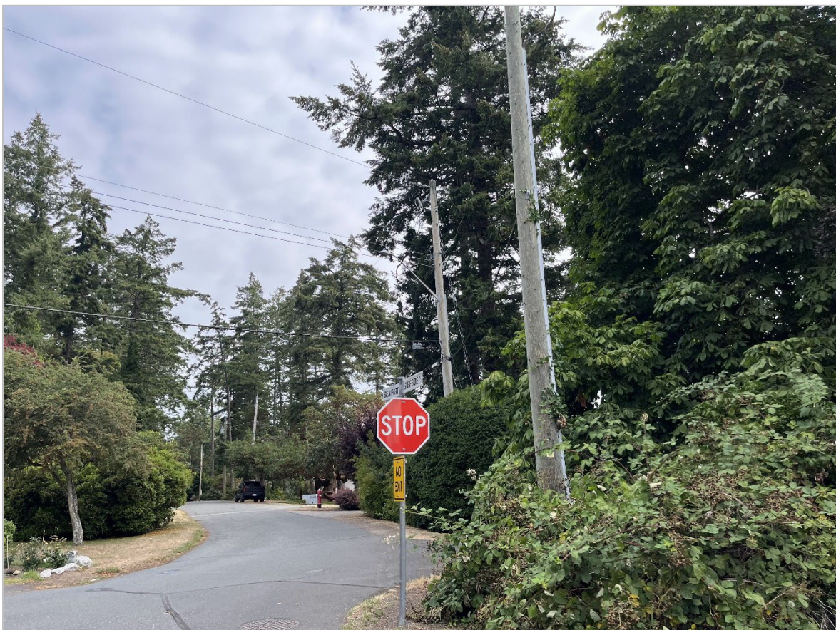
Photo 5. Overhead distribution lines are used throughout Sidney to provide electricity.
