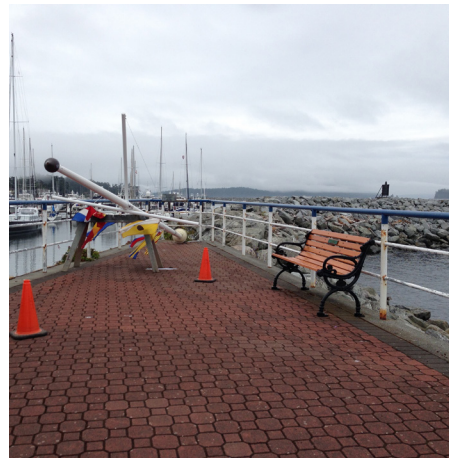
Aging infrastructure and disjointed seating elements.
