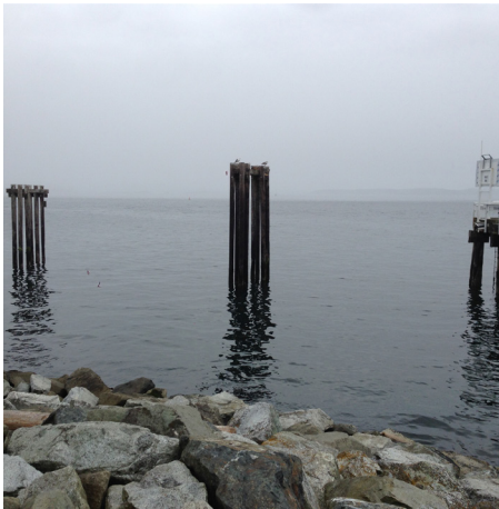
Piles that held the currently decommissioned Alpine (Sidney Spit) ferry dock.
