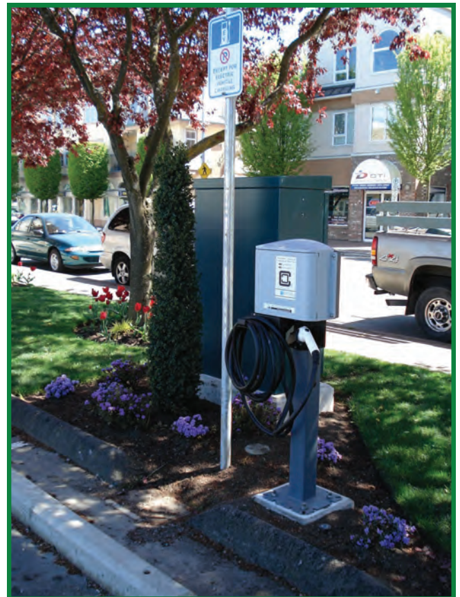
The Electric Vehicle Charging Station at Parking Lot F on Third Street
