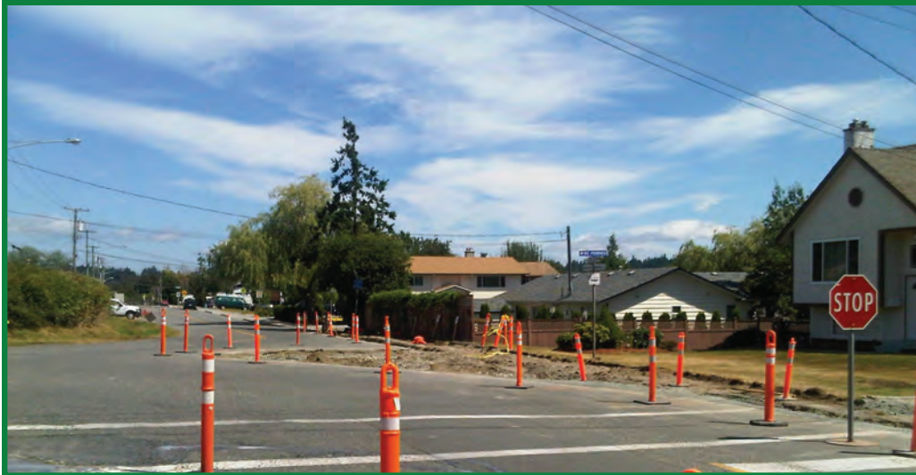
Road, curb, and sidewalk construction at McDonald Park Road and Ardwell Avenue intersection
