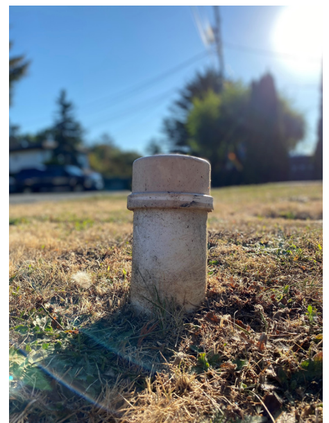
Outdoor cleanouts make it easy for professionals to access and inspect your pipes.
